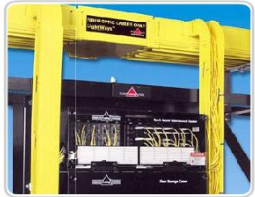
Fiber Cable Raceway
